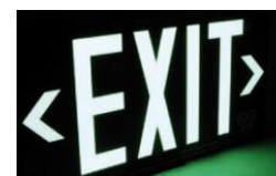
SECURITY SYSTEMS AND EMERGENCY LIGHTING
